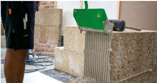
7 Glue the vertical surface in case the blocks don't have tenon and mortise joints.
