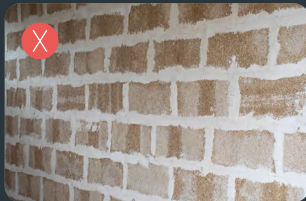
Bad joint treatment
