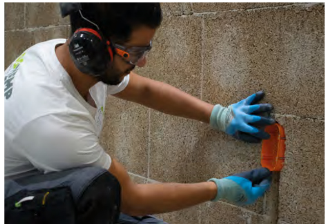
4 Collect the waste from your hemp block cuttings and grind it. Then mix it with ProKalk binder at a 50/50 ratio. Moisten the resulting mixture with water to obtain a homogeneous, slightly moist mixture. Fill the cavities with the mixture.
