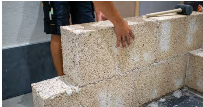
8 Place the blocks on the adhesive mortar for masonry in 3 mm slim joints.
